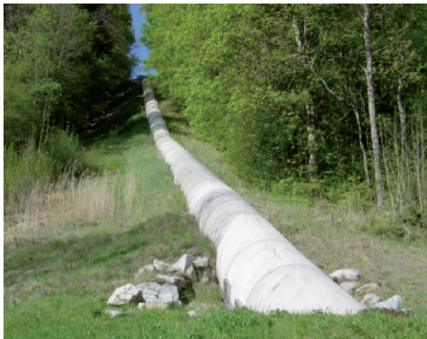
Figure II.4.21. Example of a partially buried penstock
