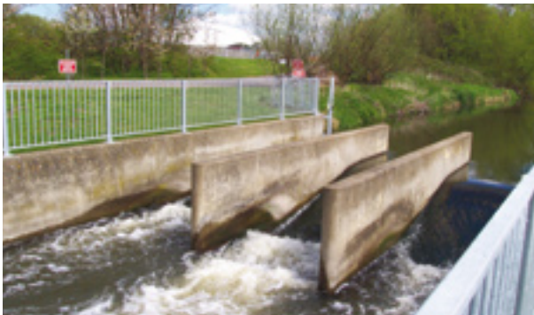
Figure I.7.15. River Colne at Berrygrove. South East England. Compound crump weir.
