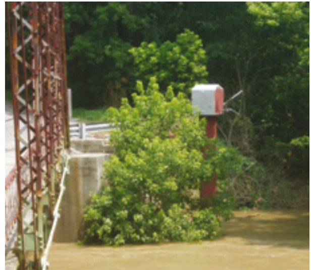
Figure I.4.4. Steel pipe stilling well and shelter attached to bridge wingwall
