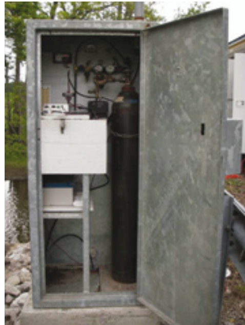
Figure I.4.9. Instrument shelter located on a stream bank
