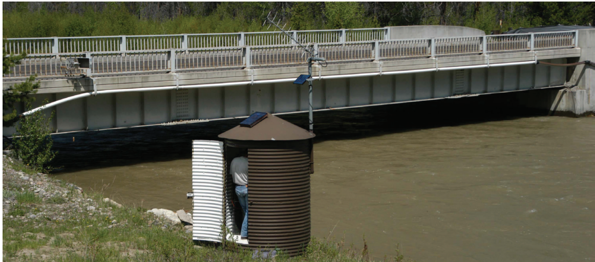
Figure I.2.1. Gauge with walk-in shelter, solar panels, satellite antenna, and wire-weight gauge on bridge
