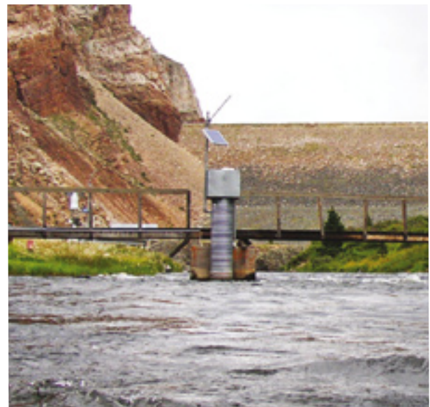
Figure I.4.5. Corrugated steel pipe stilling well and shelter attached to bridge pier
