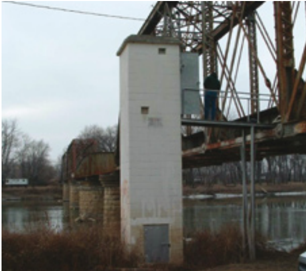
Figure I.4.3. Concrete block stilling well and shelter
