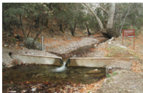
Figure I.3.5. A concrete, broad-crested artificial control with a shallow V notch in the centre
