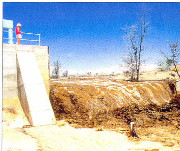
The Department of Water Affairs measures flood discharge at a number of stations along the western rivers. This is usually done via automatic recorders, such as the one housed in the blue box atop this concrete weir in the Kuiseb River downstream of Gobabeb. These data are essential if Namibia is to sustainably manage its scarce water resources.
