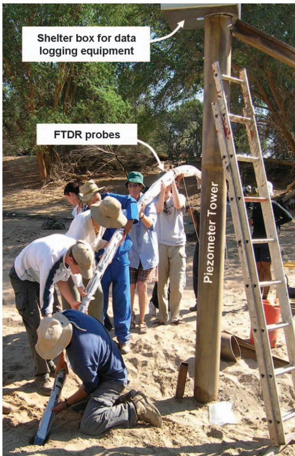
Figure 4. Installation of the FTDR probes in a slanted borehole beneath the stream channel.
